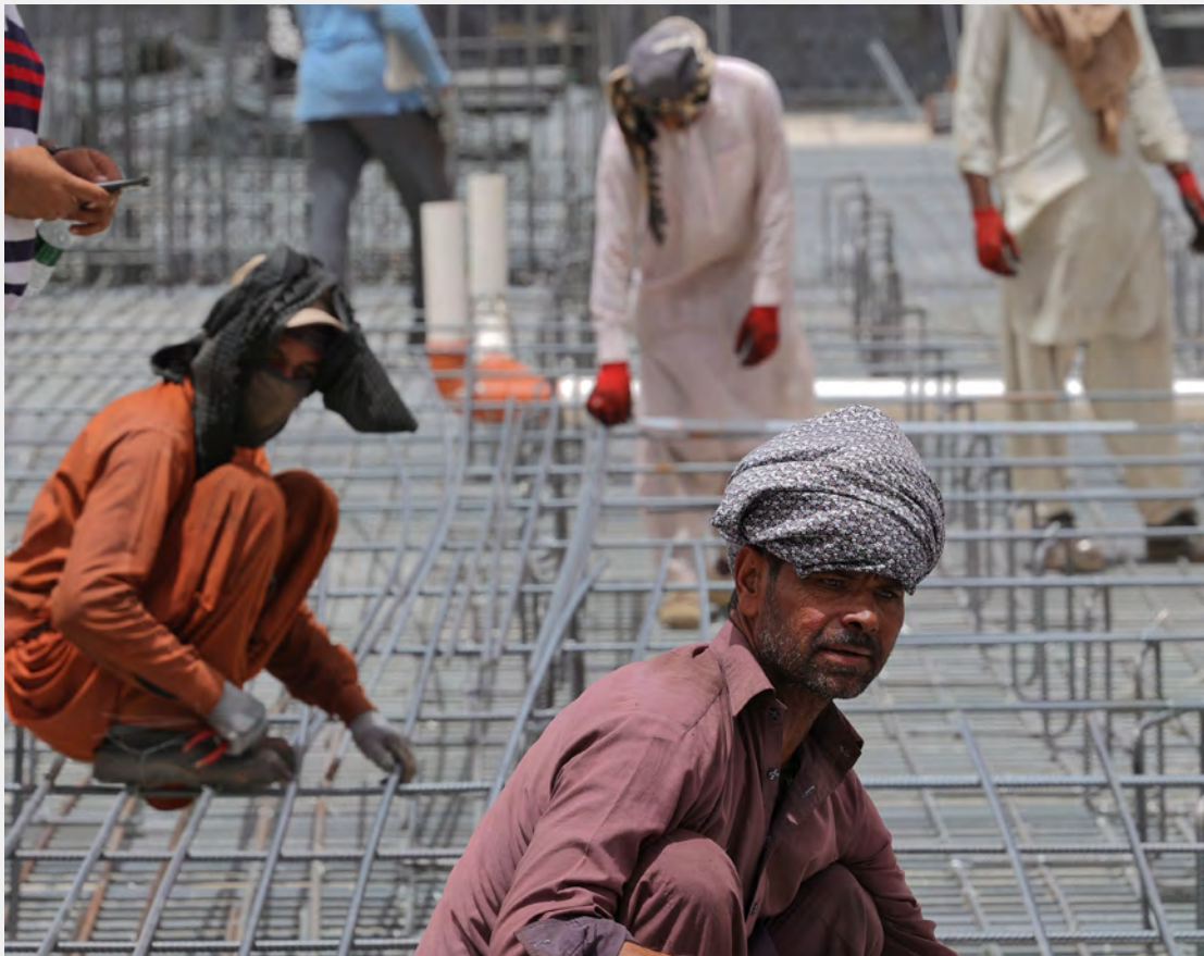
Labourers work on a steel mesh at a construction site in Saudi Arabia's capital Riyadh on May 23, 2022 during a heat wave. (Photo by Fayed Nureldine / AFP) (Photo by FAYEZ NURELDINE/AFP via Getty Images)
