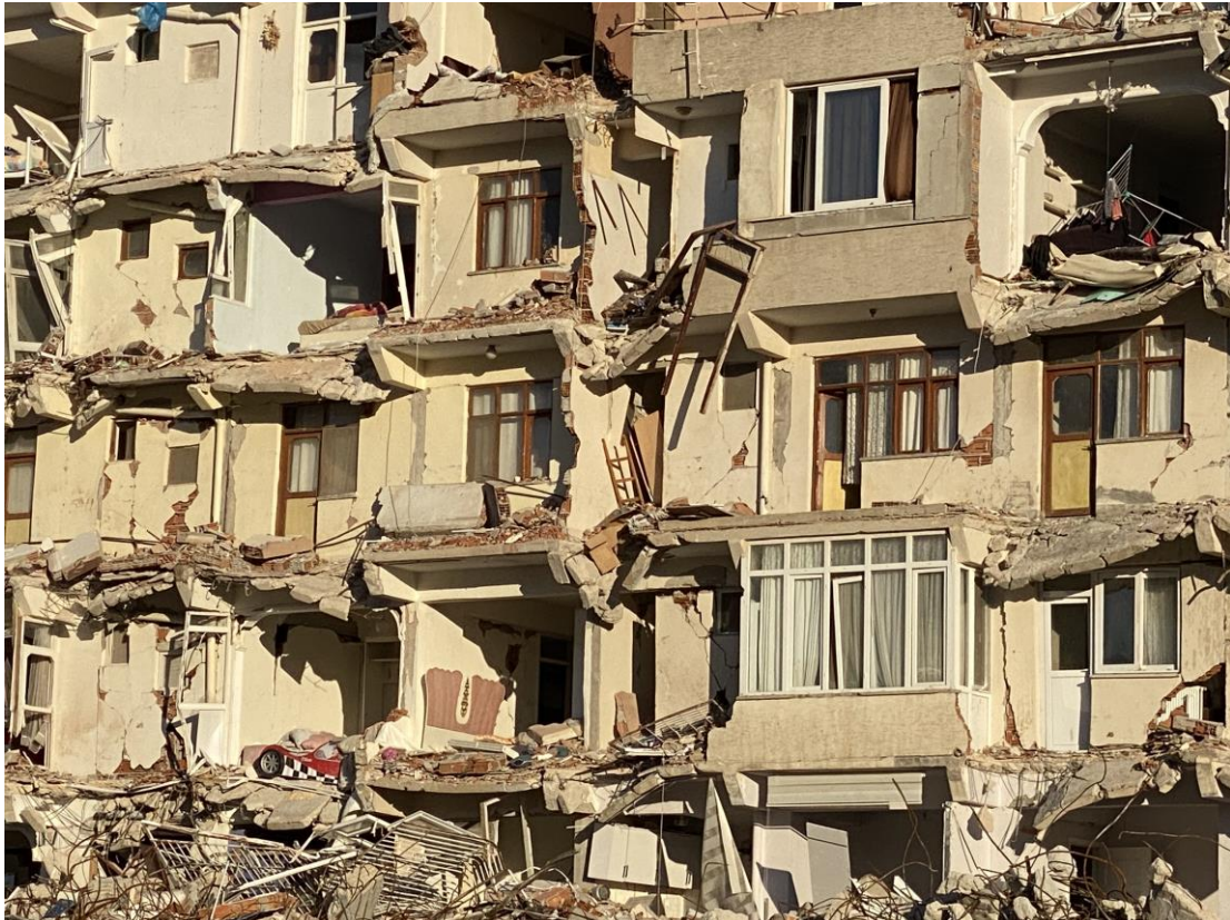
A building in Defne, Hatay province, lies in ruins. Amnesty International researchers surveyed the damage and displacement conditions in Hatay, one of the provinces most affected by the earthquakes. © Amnesty International
