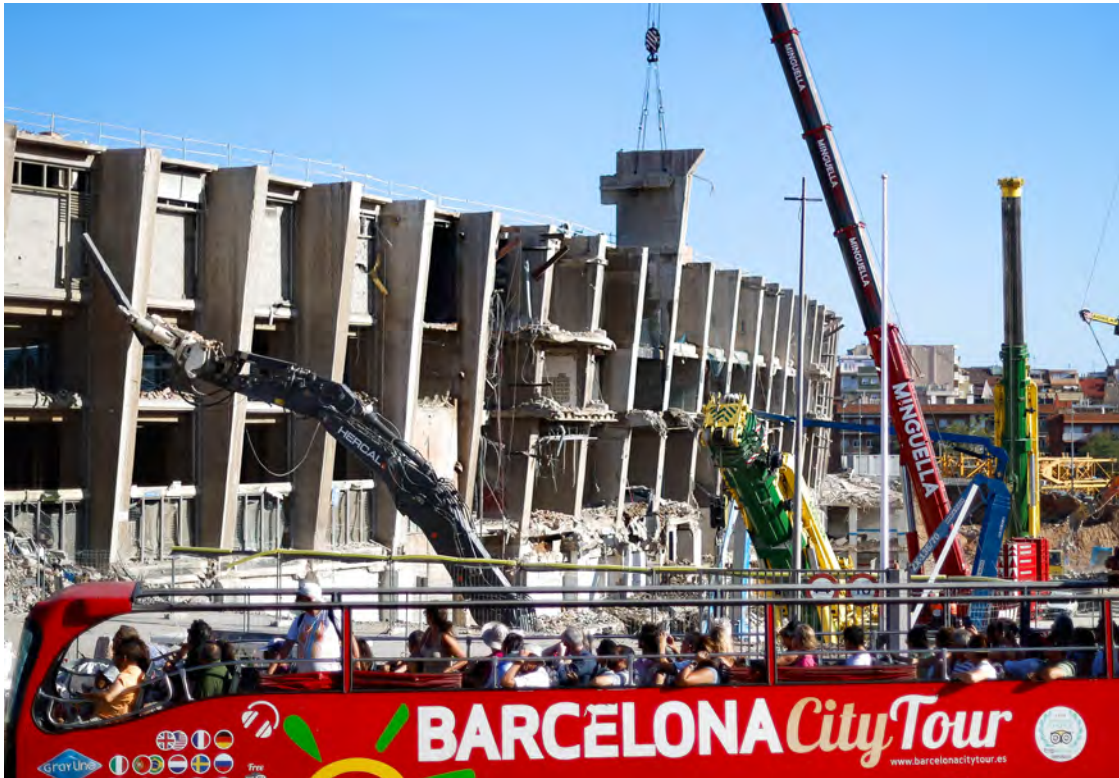
A group of tourists in a tour bus record the cranes demolishing the 3rd grandstand of the Spotify Camp Nou. The Barcelona team is renovating its stadium to expand its capacity to 105,000 spectators and will be among the most modern stadiums in the world. © Pol Cartie/SOPA Images/LightRocket via Getty Images
