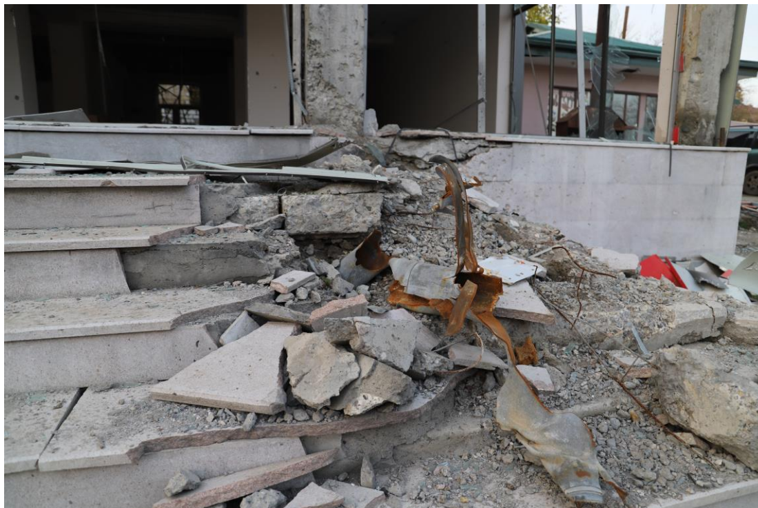
Remains of a Grad rocket fired by Azerbaijani forces embedded in the steps of a building across the road from the shop where three members of the Khachatryan family were killed in Martakert on 30 September 2020. © Amnesty International
