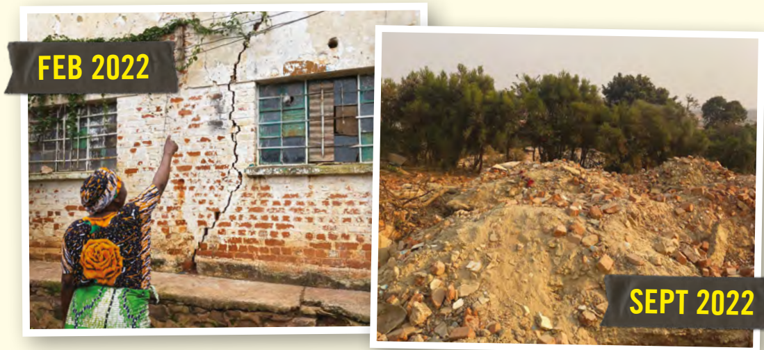
© ↑ Cécile Isaka showing crack in her house caused by the activities of the Kolwezi copper and cobalt mine operated by COMMUS, February 2022 (left); Ruins of Cécile Isaka’s house, September 2022 (right) © Amnesty International (photographer: Jean-Mobert Senga)
